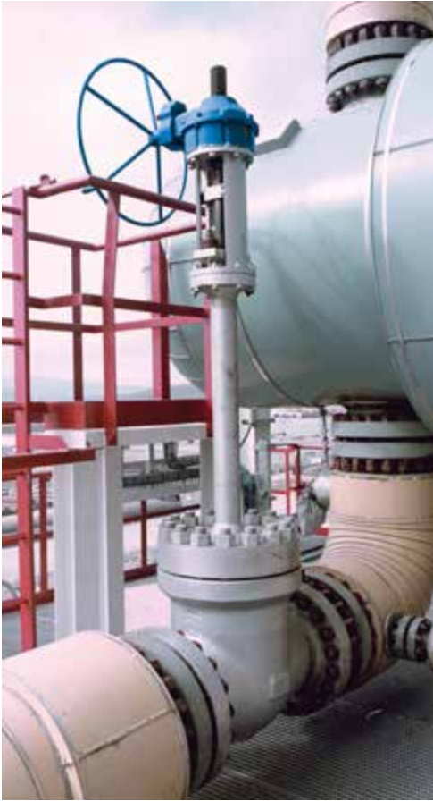
A Velan cryogenic gate valve in service.
