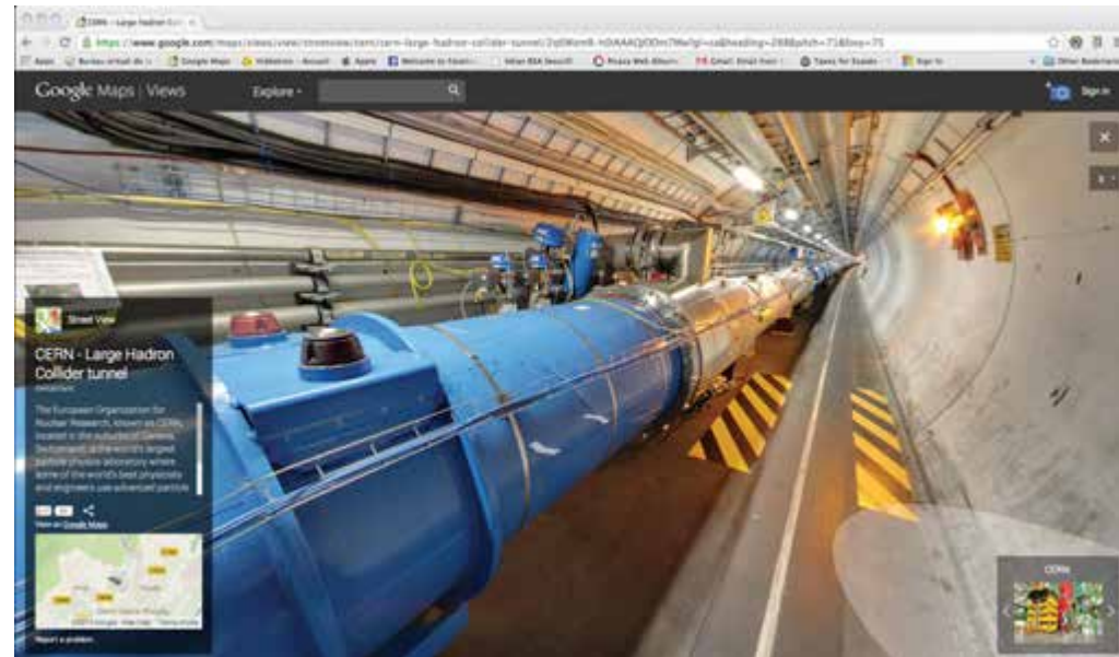
The LHC tunnel where Velan valves are installed.
